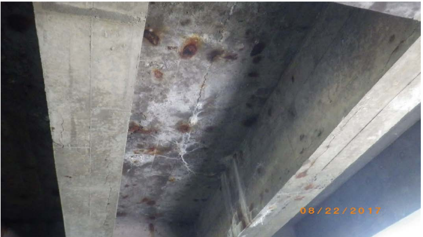
Recurring efflorescence on a beam that was patched in a rehabilitation project in 2014.
