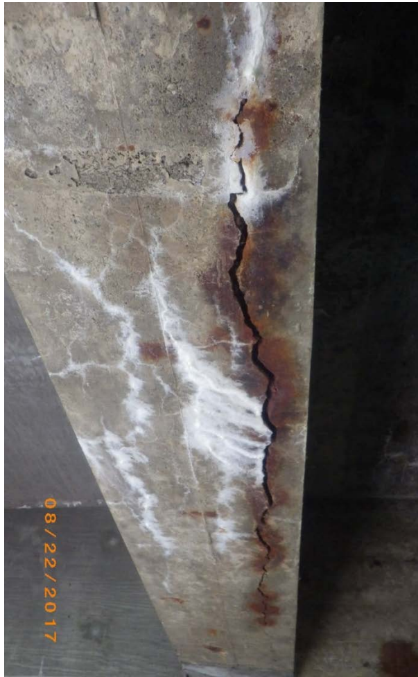
Beam cracking and efflorescence on soffit.
